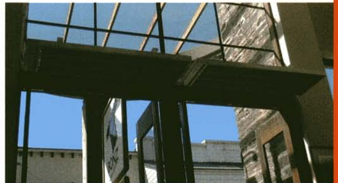
Two EnergoStrip heaters provide an effective "radiant curtain" over the main entrance to this Queenstown retail outlet.
